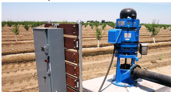
Above Photo: Electric motor powering an agricultural irrigation pump.
