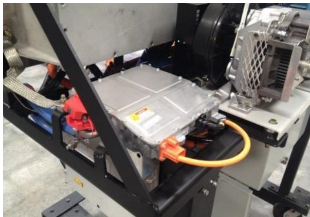
Figure 17. Close-up view of the DC-to-DC converter installed into PCAS assembly.
