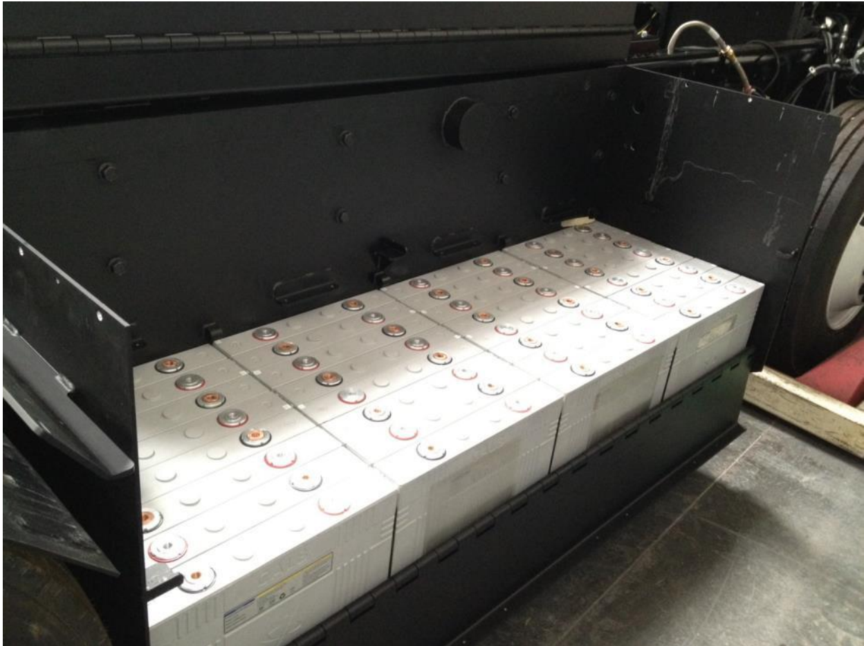
Figure 6. Photo of cells in upper compartment of new battery enclosure design.
