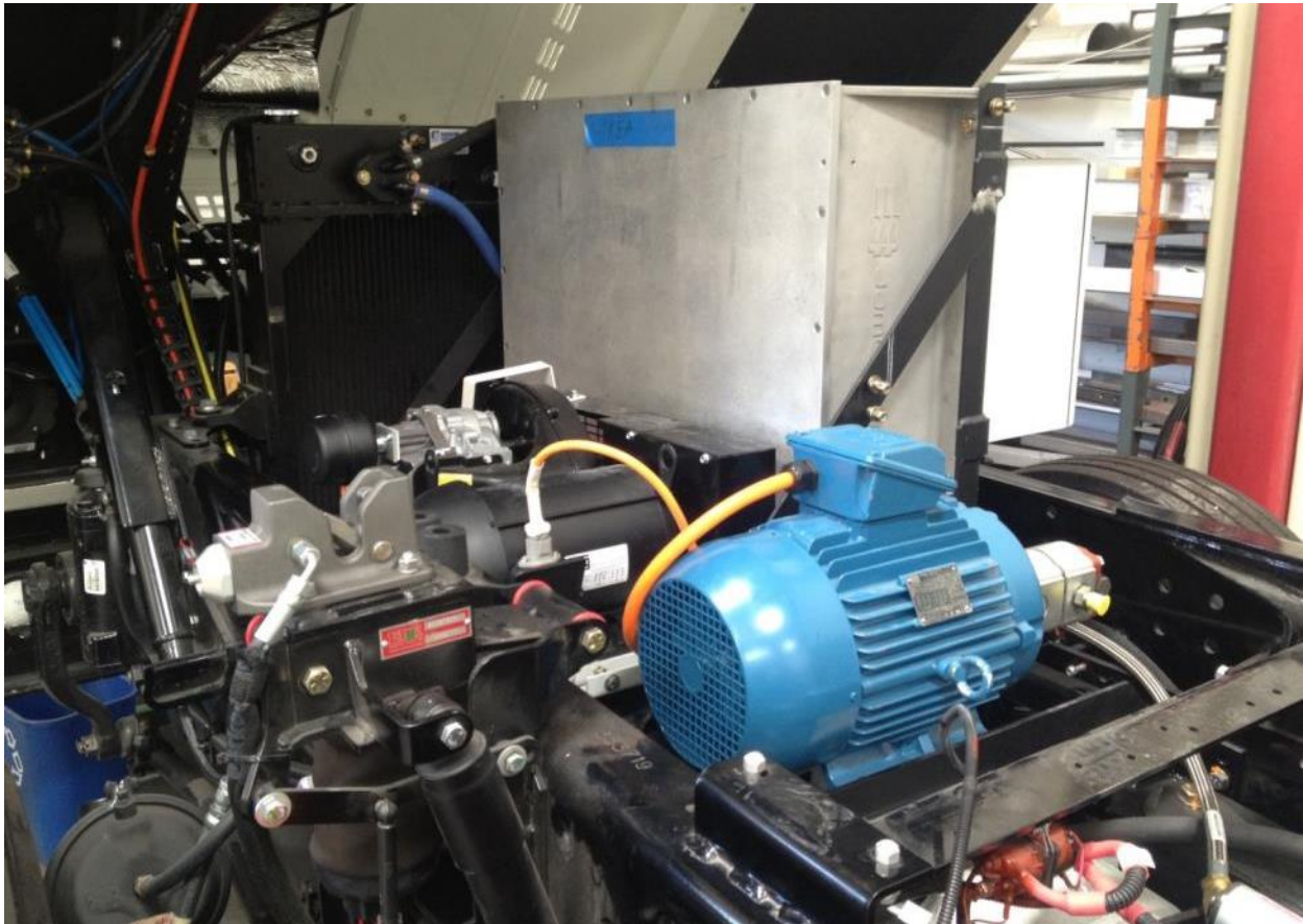
Figure 13. PCAS assembly installed in IKEA tractor.
