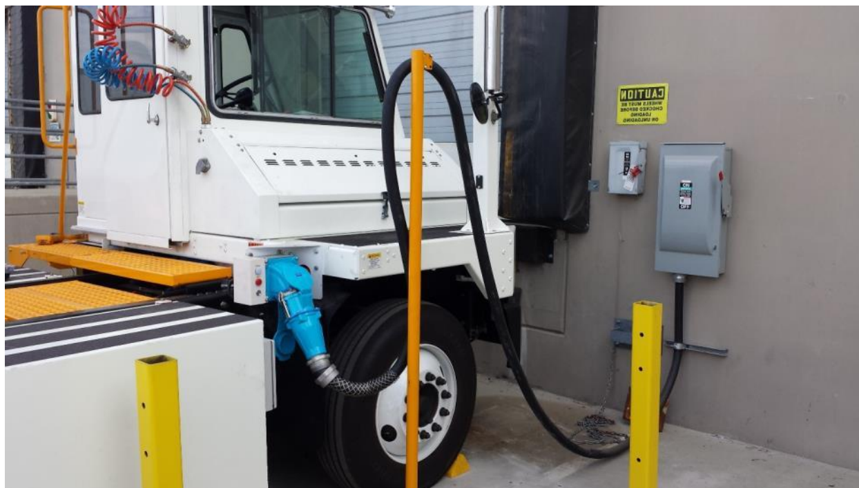
Figure 24. IKEA Tractor parking and charging infrastructure.
